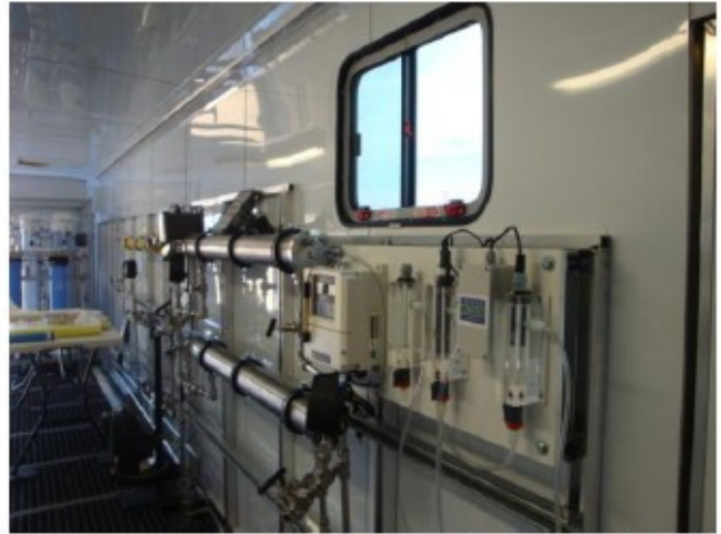
Interior of unit, set up for membrane modules
